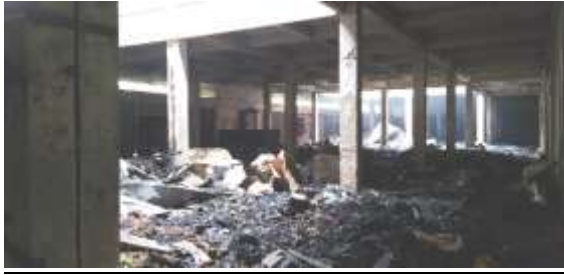
Figure 6. Condition of the Market After the 2020 Fire. Source: Regional Market Technical Implementation Unit I, Department of Industry and Trade, Banyumas Regency
